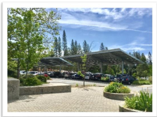
Completed installation of the solar arrays at the Eric Rood Administration Center in Nevada City, CA.
